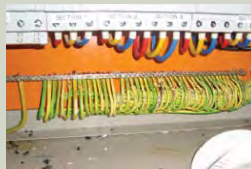
Fig2. Rat damaged electric wire (Dinesh, NPC)
