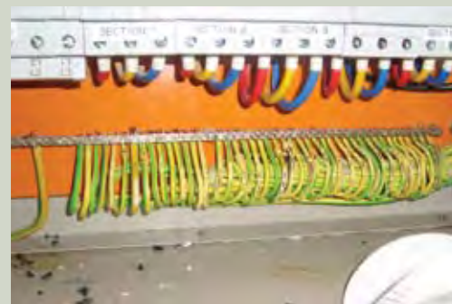
Fig2. Rat damaged electric wire (Dinesh, NPC)
